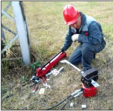
In photo PN100 in operation
