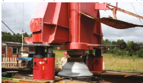
The rise of the phone tower and its holding when replacing the insulator
